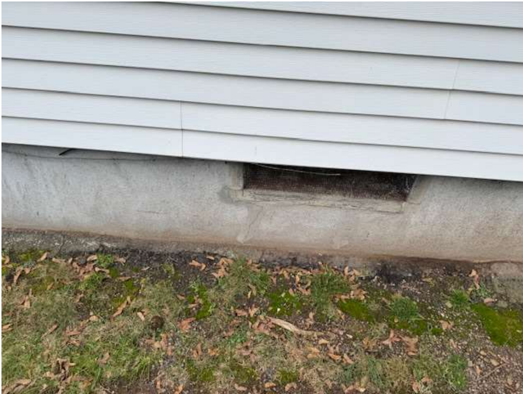
View of settlement crack in right wall.
