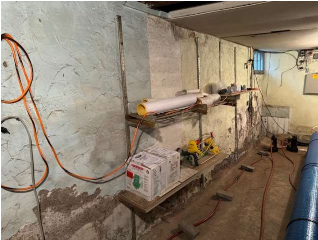
View of inside face of right wall with outward tilt.
