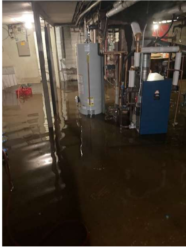
View of standing water flooding basement.
