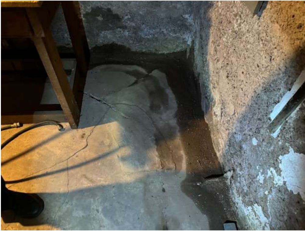
View of basement floor slab with cracking and dampness.
