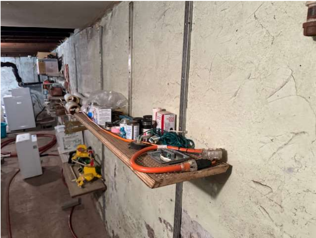
View of tilt in right foundation wall.
